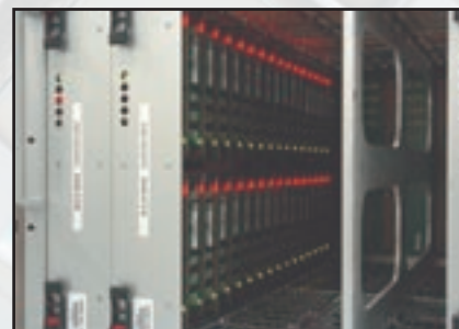
Below: Craig standing beside 12 racks
