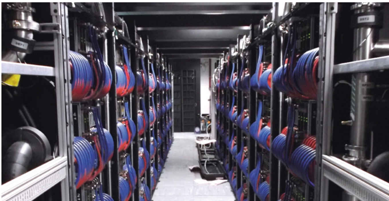
Hot and cold cooling connections to the rear of ARCHER2 compute cabinets.
