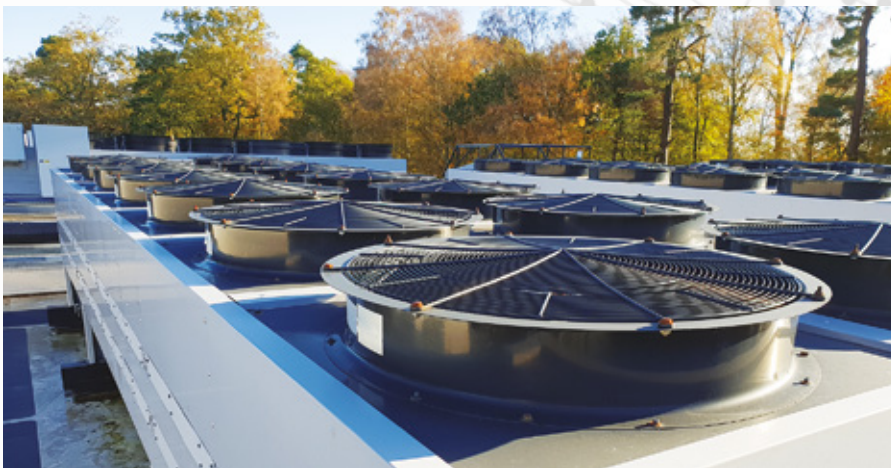
Images: (top) HPE ARCS cabinets at EPCC's Advanced Computing Facility; (lower) some of the Dry Air Cooler plant on the ACF roof which supports both the mechanical and the free cooling for Computer Rooms 2 and 3.
